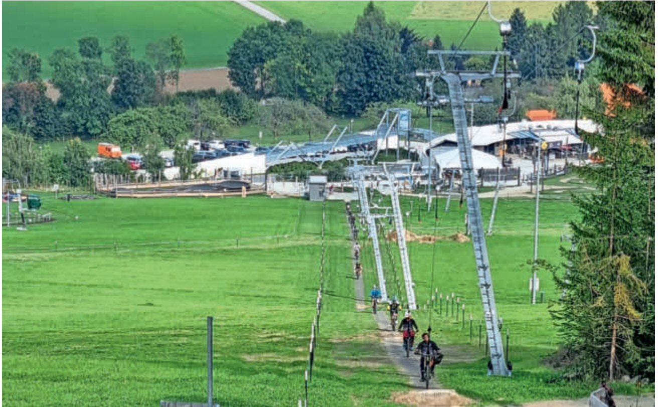
Hard-wearing grass pavers laid for regrassing and stabilization of a surface lift track
