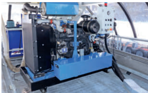
Diesel engine for the hydrostatic emergency drive in the bottom station
