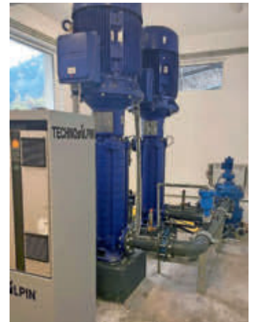
The two high-pressure pumps that feed the storage pond
