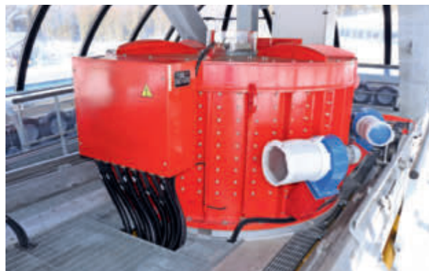
The 654 kW direct drive in the bottom station
