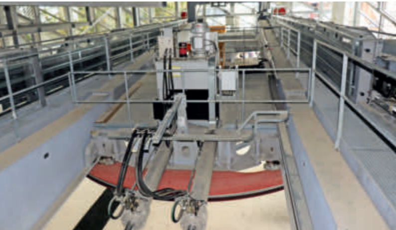
The bottom station also houses the tensioning system for the haul rope.
