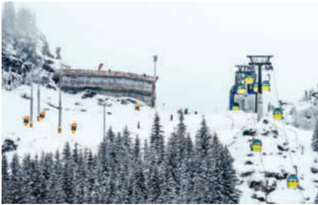
The top station and the start of the ski slope, with the future restaurant and hotel under construction on the left
