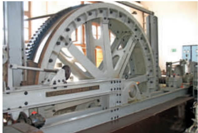
The funicular still operates with the drive train installed in 1932; in the photo, the bullwheel with two wraps of the haul rope
