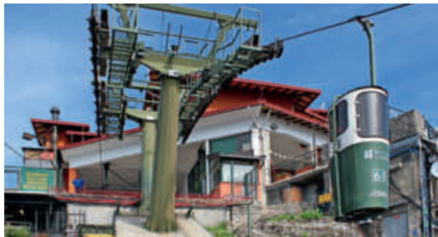
The original reinforced concrete pressure frame outside the top station was replaced by two steel-plate towers with polygonal shafts.
