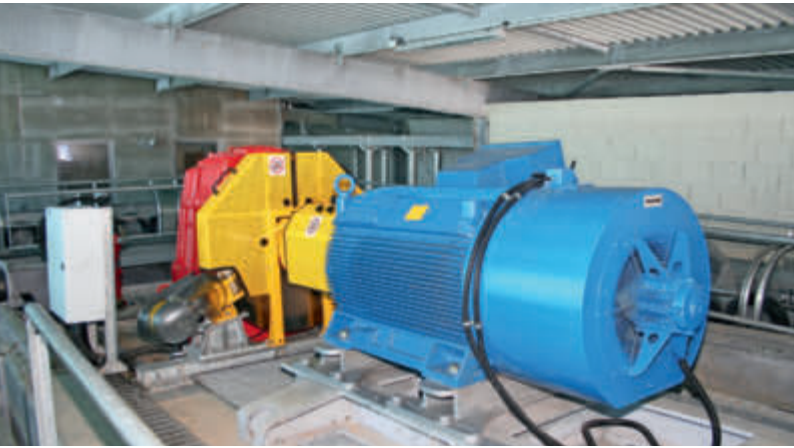
Hydraulic tensioning is used for the drive platform and bullwheel in the bottom station.
