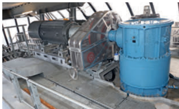
A classic electric drive with gearbox is located in the top station of the 6-seater chairlift.
