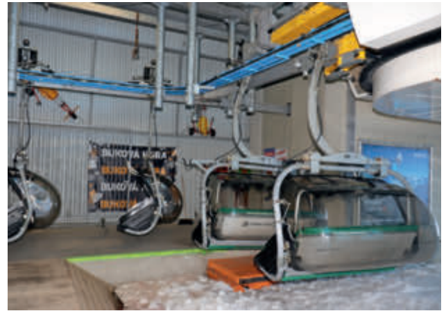
Semi-automatic parking for the chairs in the bottom station
