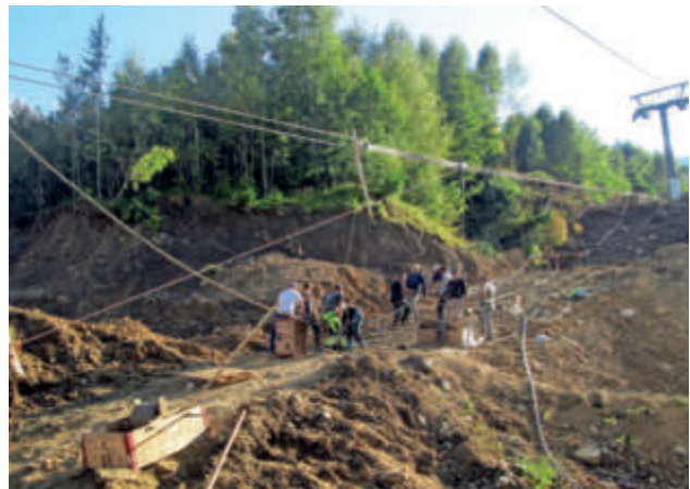
After ten years of construction work, the carrying-hauling rope was finally spliced.
