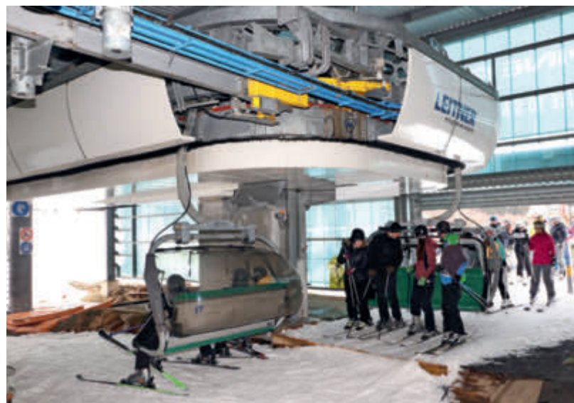
Ninety degree loading in the bottom station
