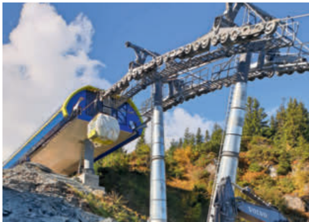
Earthworks for the ski trail in the area of the top station
