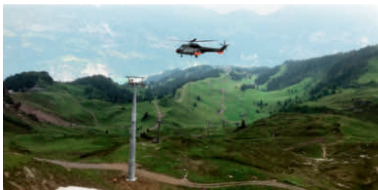
Within only two days, components with a total weight of around 340 tons were airlifted by the TH06 Super Puma transport helicopter.
