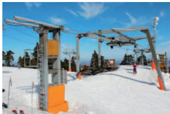
On the Dámská triple chairlift (2005 – 2019) the original counterweight system was replaced by two hydraulic cylinders for tensioning the deflection sheave.
