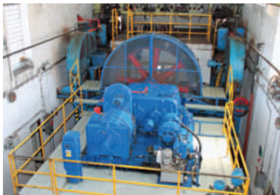
The 205 kW drive in the top station
