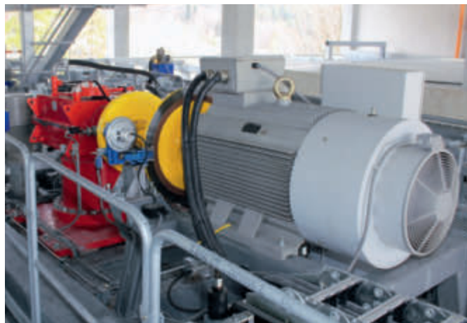
The 250 kW drive of the Beskid Sport Arena's 6-seater chairlift in Szczyrk is located in the bottom station.
