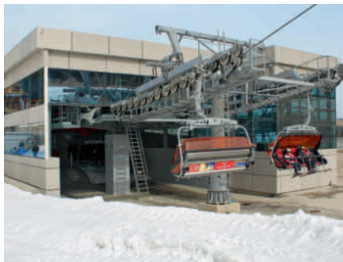
The bottom station of the Remiaszów 6-seater chairlift in Białka Tatrzańska with chair parking in a modern multipurpose building with lots of reflective glass
