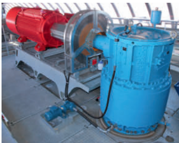
The overhead drive with 556 kW continuous output is housed in the bottom terminal.
