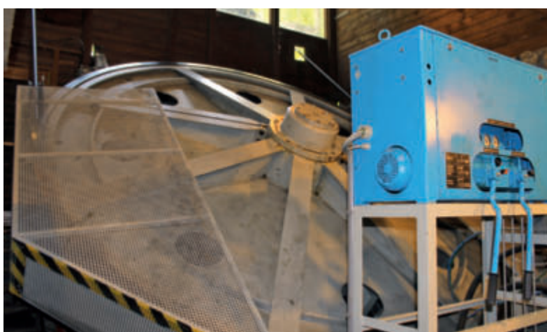
The bottom station houses the angled 4-meter bullwheel plus 45 kW d.c. motor and the hydraulic tensioning system.
