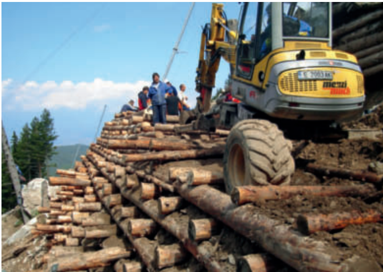
Unstable slopes were tackled with soil bioengineering methods using timber and plants instead of concrete and steel. The photo shows a log cribwall on the famous Tomba Trail.
