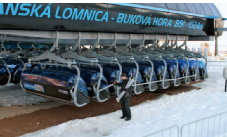
The chairs parked automatically in the lower terminal are additionally immobilized with spacer bars.
