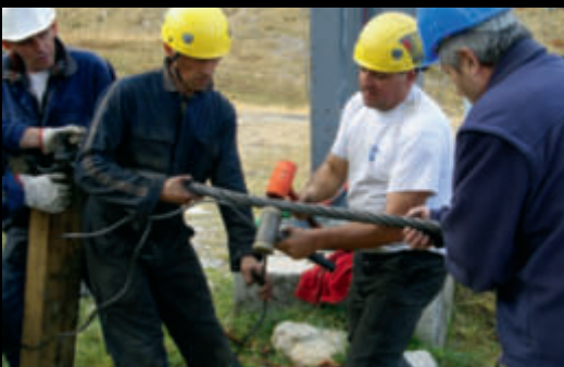
Cables and installation
