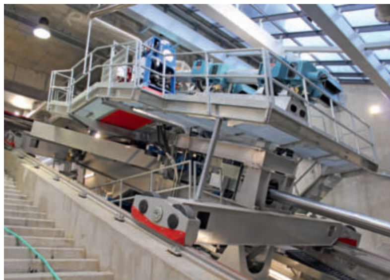
The Funitel drive, with 1,216 kN hydraulic tensioning, is angled against the inclination of the line and can be observed through the glazed roof.
